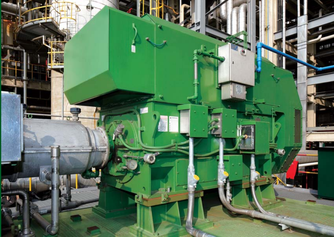
Photos: TMEIC inverter-driven Exp 4-pole, 1,900kW variable-speed induction motor and compressor
