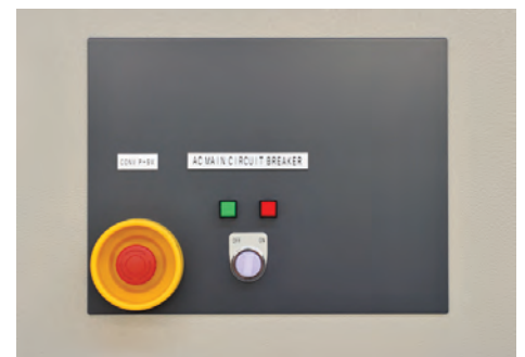
Emergency Stop Button and Circuit Breaker Operation Panel
